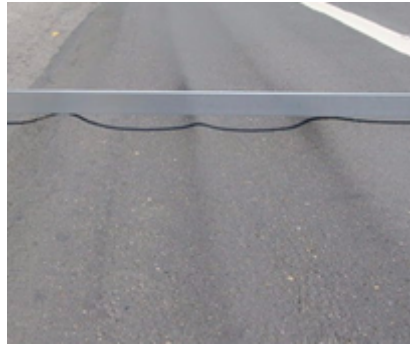
Figure 1. Image of an asphalt layer with rutting [14]
